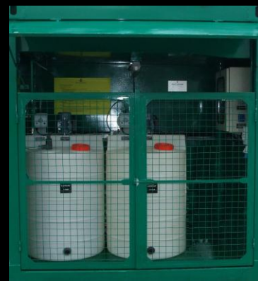
4. Security gates & hinged roof
