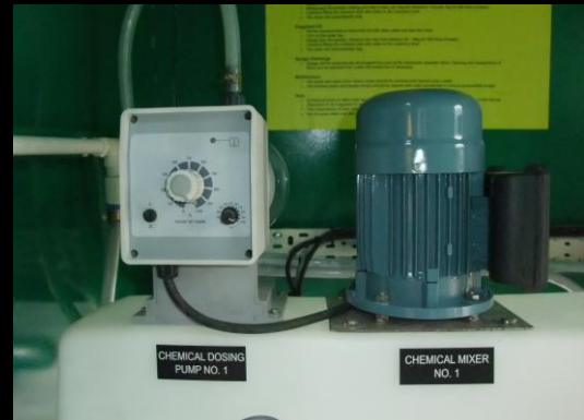
2. Automatic chemical mixing & dosing system
